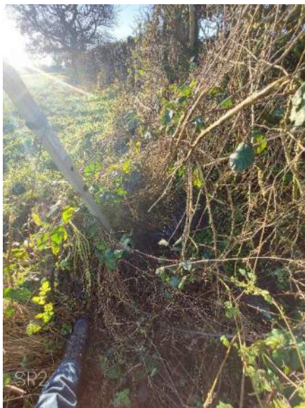
No water present. Collapsed culvert under gate.
