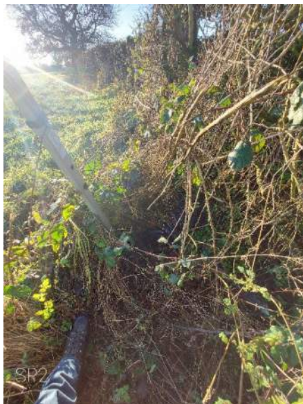
No water present. Collapsed culvert under gate.
