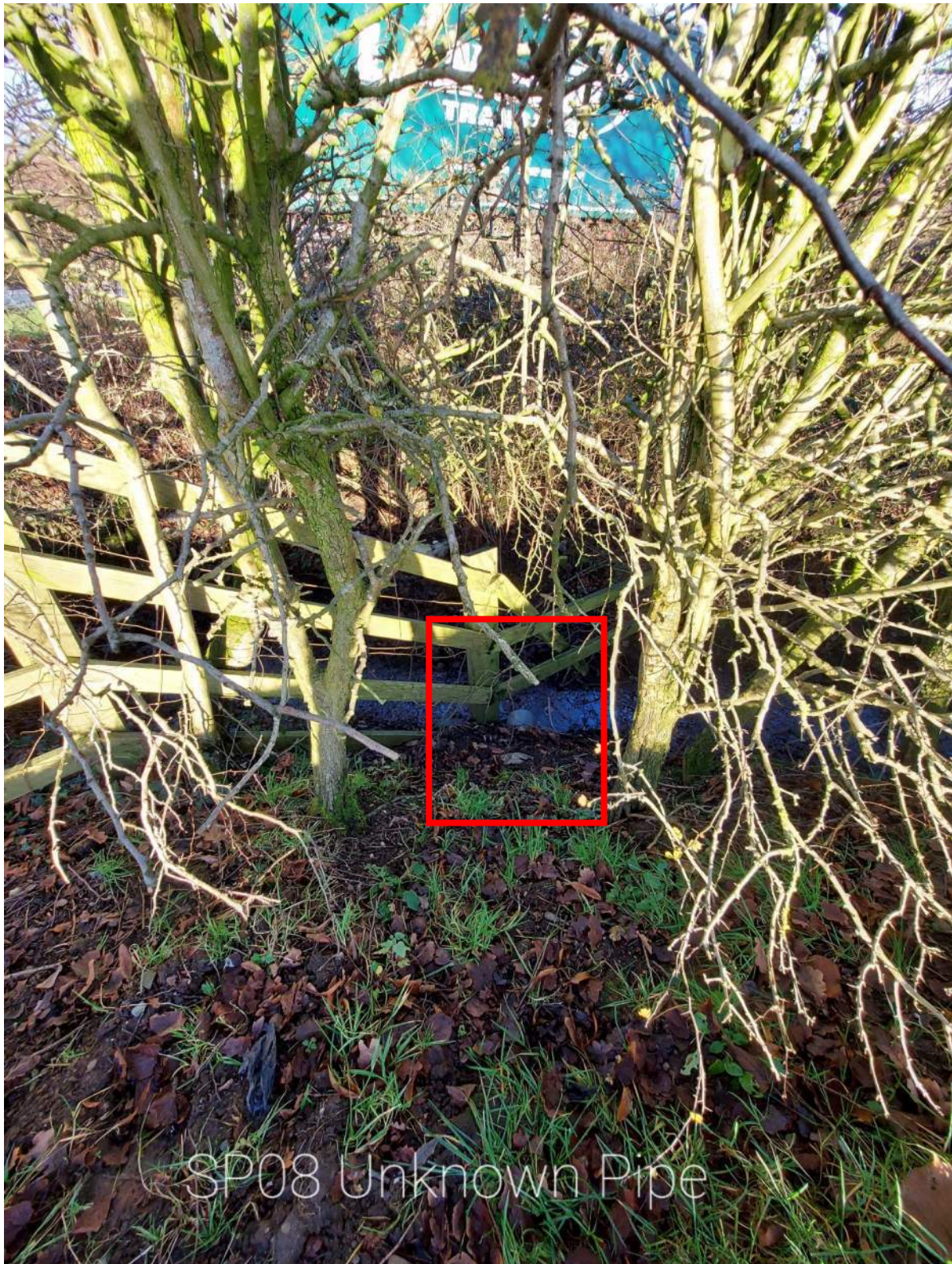
Unknown pipe found out falling into SP 08 ditch. The pipe carried constant flow with the head of the pipe unfound. Assumed to be land drainage. Exposed vertical open pipe found in the field upstream of discovered pipe (See vent pipe 02 image and General arrangement for location).
