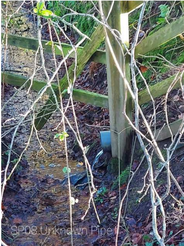
Continuous flow visible of unknown pipe.
