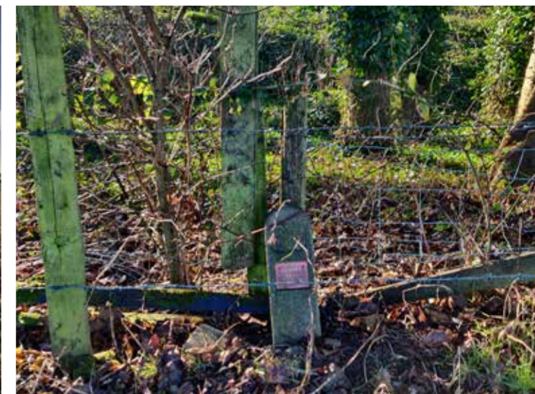
High Voltage Cable Marker by Lydiate Quarry Boundary. Looking South.
