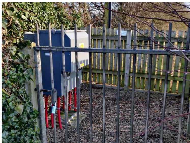
Substation 15167 adjacent to A5083 within Housing Development. Looking East.
