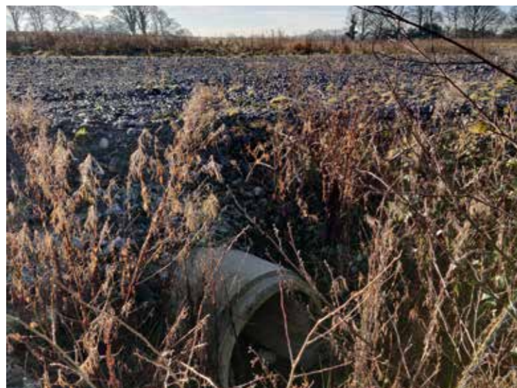
Culvert underlying Temporary Access Road to culvert leading off site. Looking Southwest.
