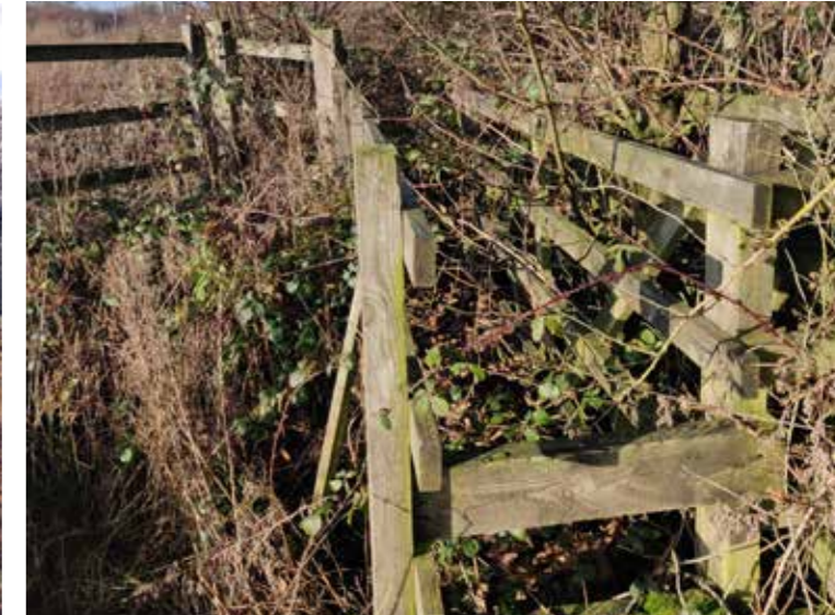
Culvert leading off site, assumed towards pond in centre of M65.A6 Roundabout. Looking North.
