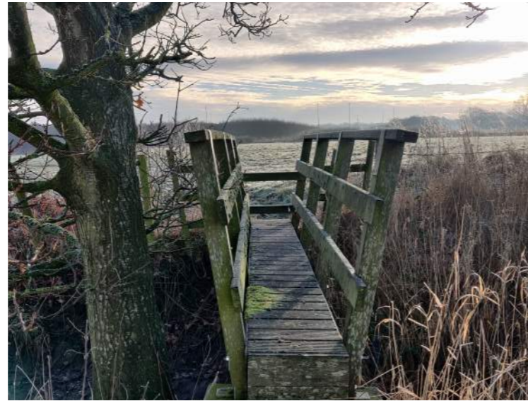
Public Footbridge from Phase A Green Infrastructure to Phase A. Looking East.
