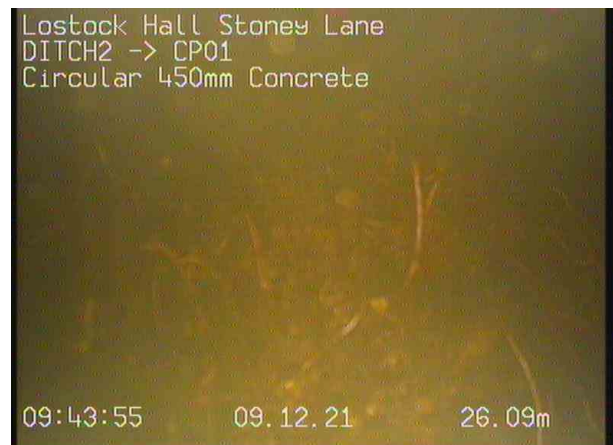
DITCH2X_652f154b-e4d7-4485-9329-7ac427e47d08_20211209_094826_618.jpg, 00:05:29, 26.09 m Roots, mass, 30% cross-sectional area loss
