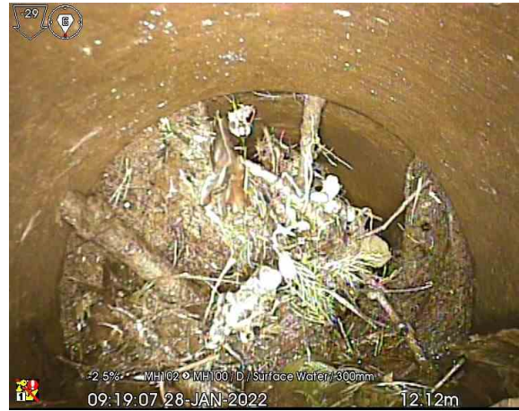
MH102X_12-12m_091907.jpg, 00:01:54, 12.12 m Roots, mass at joint, 70% % cross-sectional area loss
