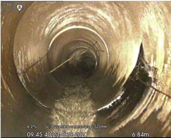
MH105X_6-84m_094540.jpg, 00:00:43, 6.84 m Roots, fine at joint
