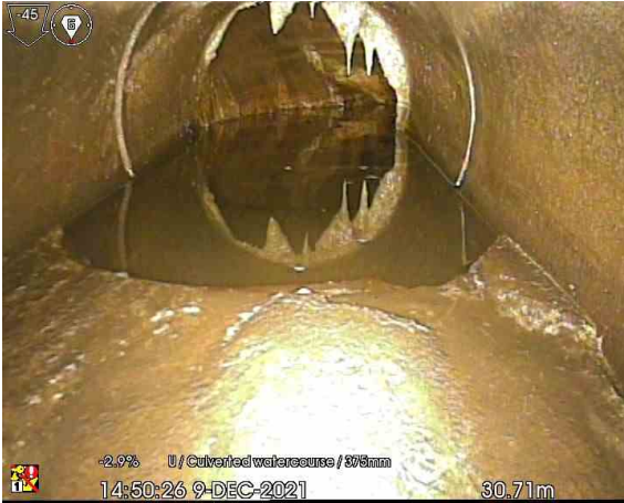
DITCH6 PIPE A_30-71m_145026.jpg, 00:02:27, 30.71 m Survey abandoned, Unable to drive over concrete
