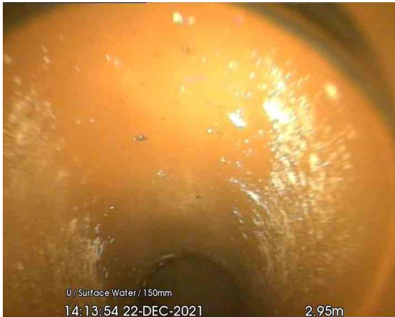
CP3X_2-95m_141354.jpg, 00:00:18, 2.95 m Joint displaced, medium
