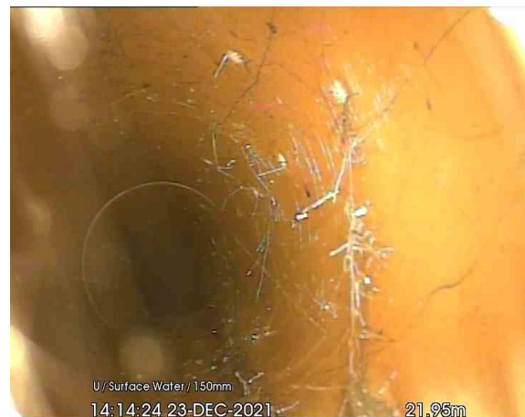
CP3 PIPE A_21-95m_141424.jpg, 00:02:14, 21.95 m Roots, fine
