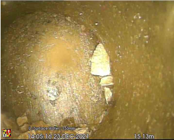
CP3 PIPE C_15-13m_140516.jpg, 00:01:32, 15.13 m Finish node type, other special chamber, reference number: PIPE C, LINE CAPPED
