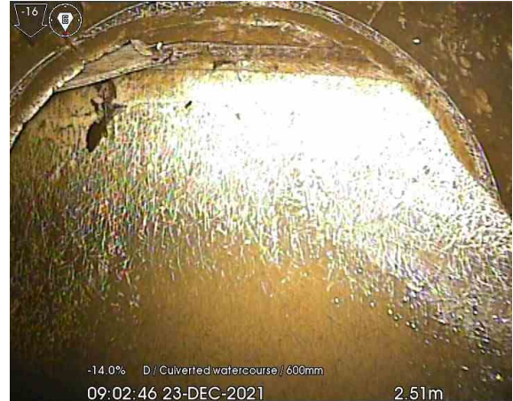
MH112X_2-51m_090246.jpg, 00:01:41, 2.51 m General photograph taken at this point, Possibly a syphon before reducing down into the outfall in the River Lostock. Dye tested to prove the connectivity.
