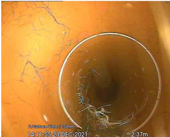
CP3 PIPE A_2-37m_141155.jpg, 00:00:22, 2.37 m Roots, fine
