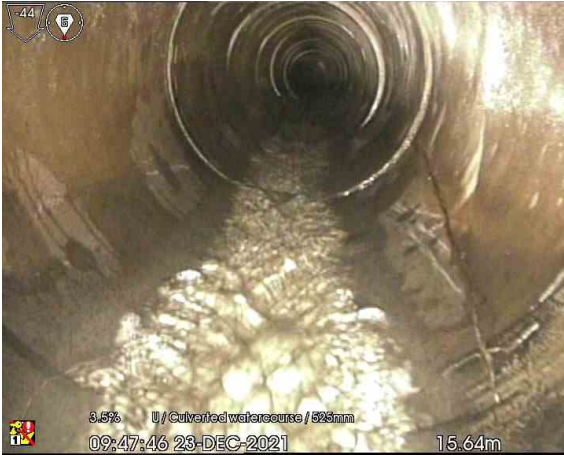
MH105X_15-64m_094746.jpg, 00:01:50, 15.64 m Roots, fine at joint
