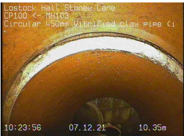
CP100X_0b6959cb-bf47-4b35-be67-4c037a8aafa6_20211207_092744_477.jpg, 00:03:38, 10.34 m Joint displaced, medium
