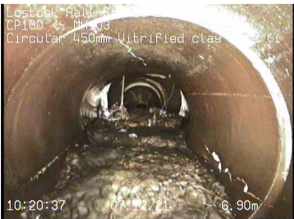
CP100X_a968e610-510b-4e61-b553-cfb58d9e4c08_20220105_074449_126.jpg, 00:01:18, 6.90 m Fracture, longitudinal at 4 o'clock
