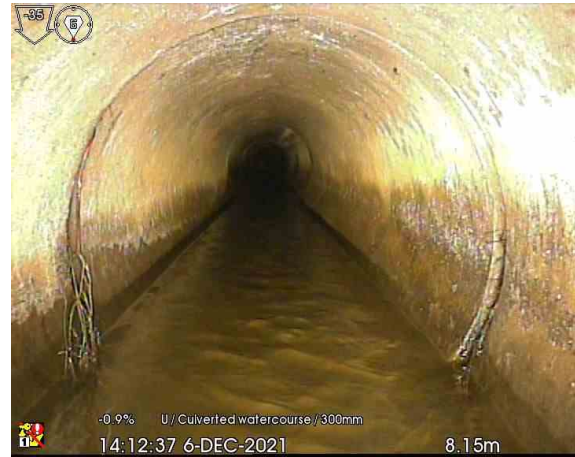
MH102X_8-15m_141237.jpg, 00:01:06, 8.15 m Roots, fine at joint
