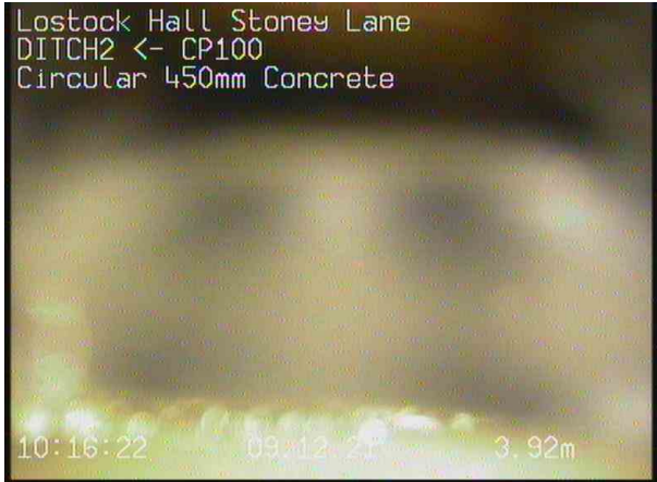
DITCH2X_b0d974d4-ab85-4ca4-95ce-bd05c55802fc_20211209_102053_454.jpg, 00:01:55, 3.92 m Survey abandoned, Unable to pass mass roots. Robotic cutter needed. Unable to remove with Warthog. Survey Overlapped.
