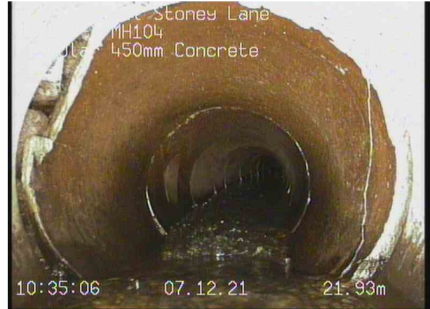
MH103X_3b172e0e-65d9-4f6a-8d7d-240340eeaa79_20211207_093854_396.jpg, 00:02:12, 21.93 m Hole in drain or sewer at a joint from 9 o'clock to 11 o'clock
