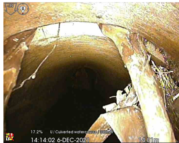
MH102X_14-01m_141402.jpg, 00:02:07, 14.01 m Survey abandoned, Unable to pass mass roots. Line needs root cutting. TM Needed.
