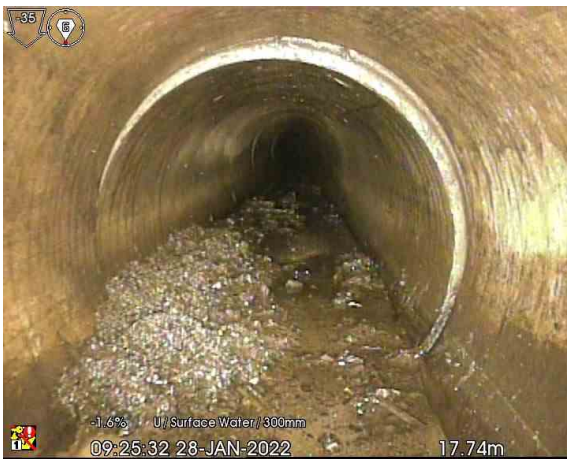
MH102 Upstream_17-74m_092532.jpg, 00:02:09, 17.74 m Settled deposits, fine, 25% % cross-sectional area loss
