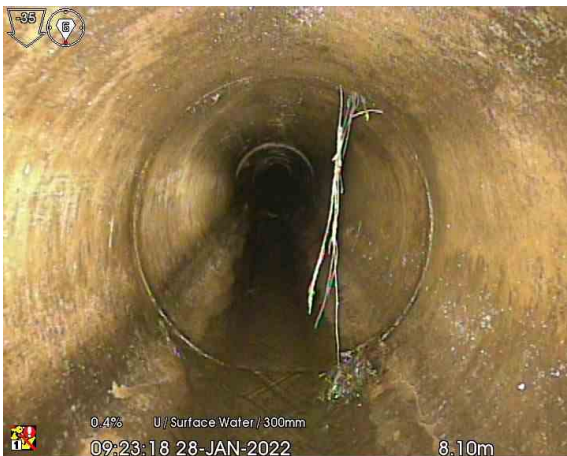
MH102 Upstream_8-10m_092318.jpg, 00:00:44, 8.10 m Roots, fine at joint
