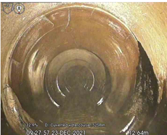
MH106X_12-64m_092757.jpg, 00:01:29, 12.64 m Cracks, multiple at joint, from 08 to 04 o'clock
