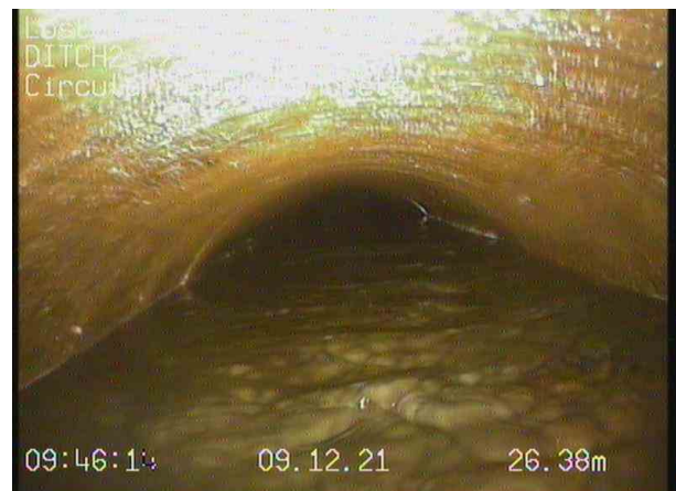
DITCH2X_af5a118b-9635-4d59-94f7-40bb4923ea76_20211209_095044_894.jpg, 00:07:05, 26.37 m Survey abandoned, Unable to remove mass roots with warthog. Needs a robotic cutter. Survey Overlapped from CP01
