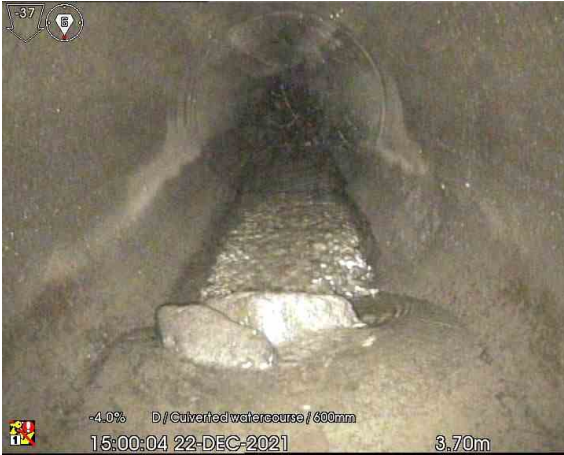
MH109X_3-70m_150004.jpg, 00:00:20, 3.70 m Other obstacles in invert, from 05 to 07 o'clock, 10% % cross-sectional area loss, Rock
