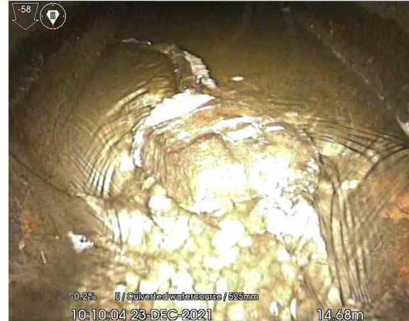
MH104X_14-68m_101004.jpg, 00:01:30, 14.68 m Other obstacles in invert, from 05 to 07 o'clock, 10% % cross-sectional area loss, Rock
