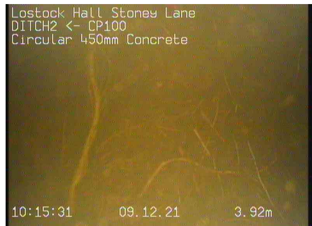
DITCH2X_893ca743-d2f4-4384-ab6f-36db9748845d_20211209_102002_264.jpg, 00:01:32, 3.92 m Roots, tap
