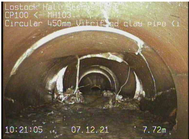
CP100X_f25e2b2b-5fe8-4ce4-9d80-9e239a8192aa_20211207_092453_375.jpg, 00:01:44, 7.72 m Fracture, multiple at joint from 12 o'clock to 12 o'clock
