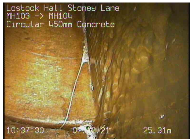
MH103X_62b509ee-8da6-429a-a5f8-ef328ec179a6_20211207_094118_056.jpg, 00:04:10, 25.31 m Crack, longitudinal at joint at 7 o'clock
