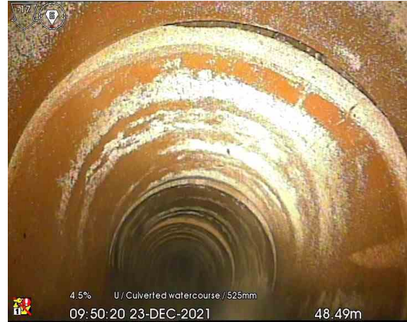
MH105X_48-49m_095020.jpg, 00:04:16, 48.49 m Open joint, medium
