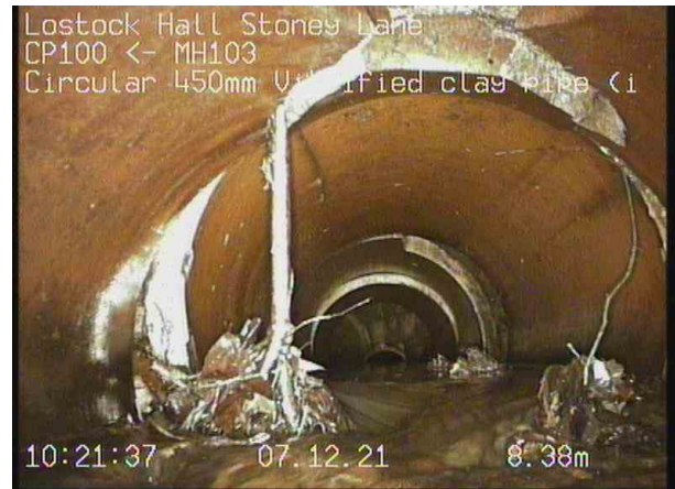
CP100X_70b78f9b-2b52-403e-a9fe-9ac17ee53f7c_20211207_092525_523.jpg, 00:02:12, 8.38 m Roots, tap at joint
