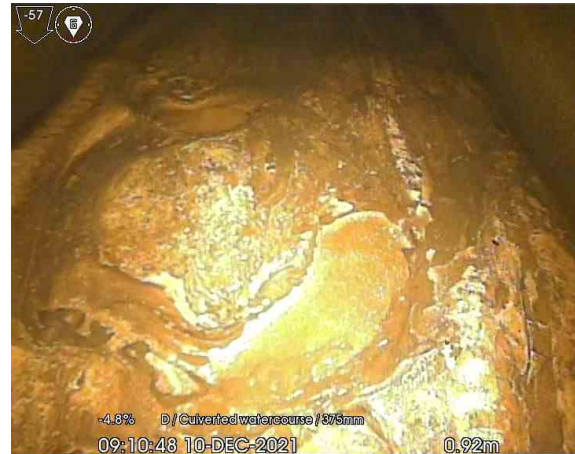
MH113X_0-92m_091048.jpg, 00:00:31, 0.92 m Attached deposits, other from 4 o'clock to 8 o'clock, 30% cross-sectional area loss, Unable to remove remaining Concrete
