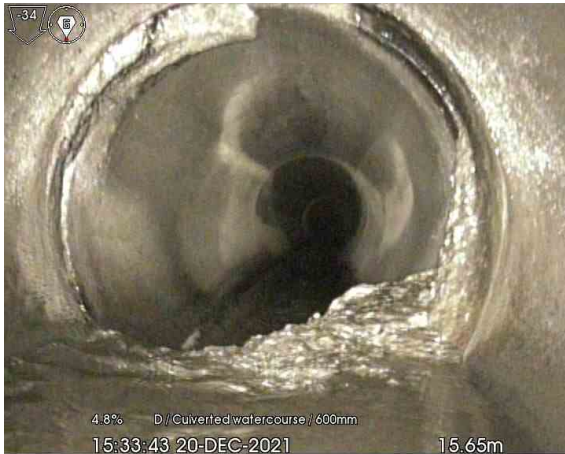
MH115X_15-65m_153343.jpg, 00:01:27, 15.65 m Attached deposits, encrustation at joint, from 03 to 07 o'clock, 15% % cross-sectional area loss
