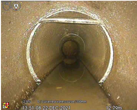
MH6X_12-79m_135108.jpg, 00:01:44, 12.79 m Sealing ring intruding, intruding but not hanging, from 10 to 02 o'clock
