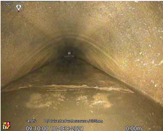
MH113X_0-00m_091000.jpg, 00:00:06, 0.00 m Attached deposits, other from 4 o'clock to 8 o'clock, 30% cross-sectional area loss, Concrete in line
