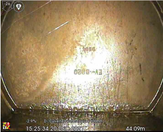
MH116Y_44-09m_152534.jpg, 00:03:08, 44.09 m Finish node type, outfall, reference number: OUTFALL, Flap valve on the outfall. Outfalls into the River Lostock.
