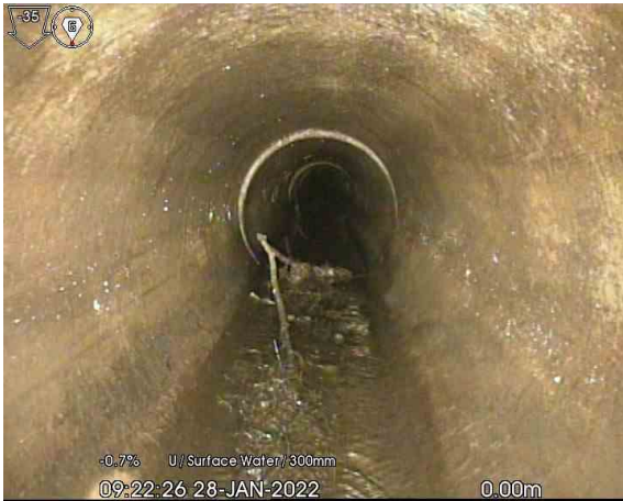
MH102 Upstream_0-00m_092226.jpg, 00:00:05, 0.00 m Roots, tap
