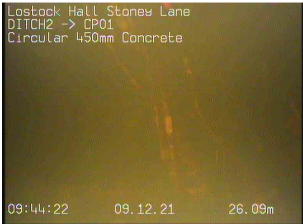
DITCH2X_91dc0210-5a83-4af4-ba15-f31d7ec9e9b7_20211209_094853_573.jpg, 00:06:01, 26.09 m Roots, tap at joint
