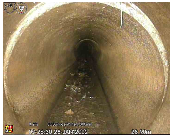
MH102 Upstream_28-90m_092630.jpg, 00:03:00, 28.90 m Settled deposits, fine, 10% % cross-sectional area loss
