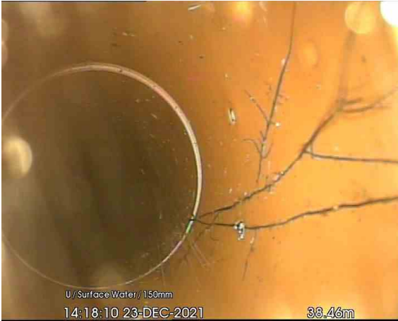
CP3 PIPE A_38-46m_141810.jpg, 00:05:32, 38.46 m Survey abandoned, Unable to push any further
