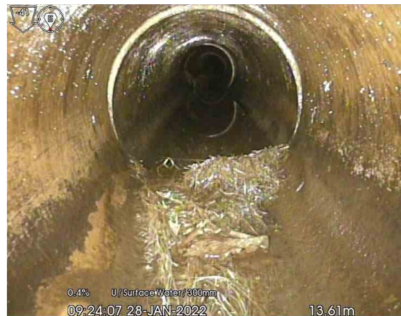
MH102 Upstream_13-61m_092407.jpg, 00:01:23, 13.61 m Roots, mass at joint, 20% % cross-sectional area loss
