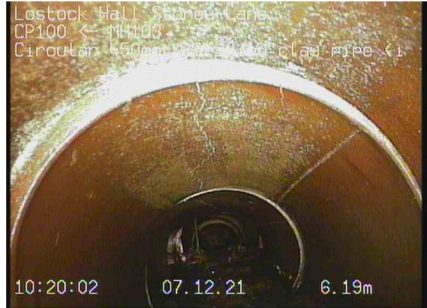
CP100X_81ea9923-0b11-4158-8616-5000123291da_20211207_092350_574.jpg, 00:01:00, 6.19 m Crack, longitudinal, in roof slab at 1 o'clock
