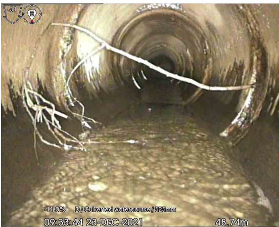
MH106X_48-74m_093344.jpg, 00:06:28, 48.74 m Roots, tap at joint
