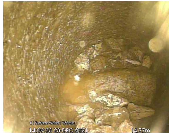
CP3 PIPE D_14-77m_140933.jpg, 00:01:20, 14.77 m Finish node type, other special chamber, reference number: PIPE D, LINE CAPPED
