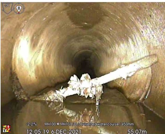
MH100X_55-07m_120519.jpg, 00:06:28, 55.07 m Other obstacles from 2 o'clock to 8 o'clock, 10% cross-sectional area loss, Bar or branch stuck in the joint
