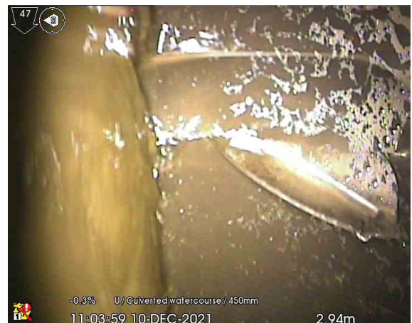
POND1X_2-94m_110359.jpg, 00:00:48, 2.94 m Infiltration, gushing, from 10 to 09 o'clock
