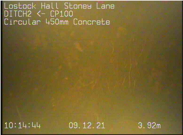
DITCH2X_d0e641f9-1ac0-4818-897b-d3a3cd028c56_20211209_101915_093.jpg, 00:00:55, 3.92 m Roots, mass, 30% cross-sectional area loss
