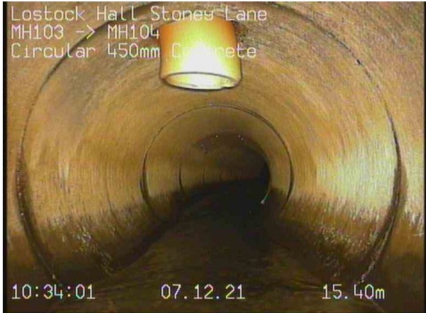
MH103X_14f17149-adf5-4275-b571-e659c8eb35b5_20211207_093749_231.jpg, 00:01:21, 15.40 m Connection defective, connecting pipe is intruding at 12 o'clock, diameter: 150mm, intrusion: 10%, GY2
