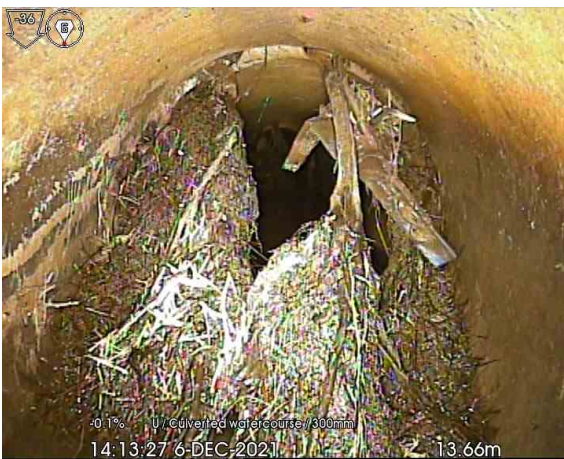
MH102X_13-66m_141327.jpg, 00:01:46, 13.66 m Roots, mass at joint, 90% % cross-sectional area loss
