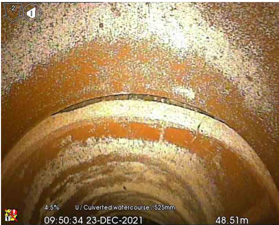
MH105X_48-51m_095034.jpg, 00:04:24, 48.51 m Soil visible beyond defect
