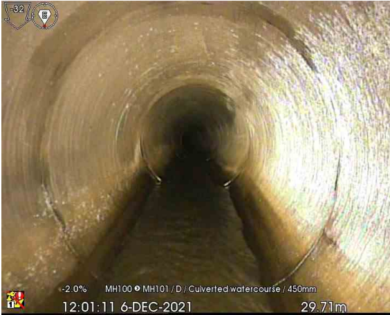
MH100X_29-71m_120111.jpg, 00:03:00, 29.71 m Crack, circumferential, at 12 o'clock
