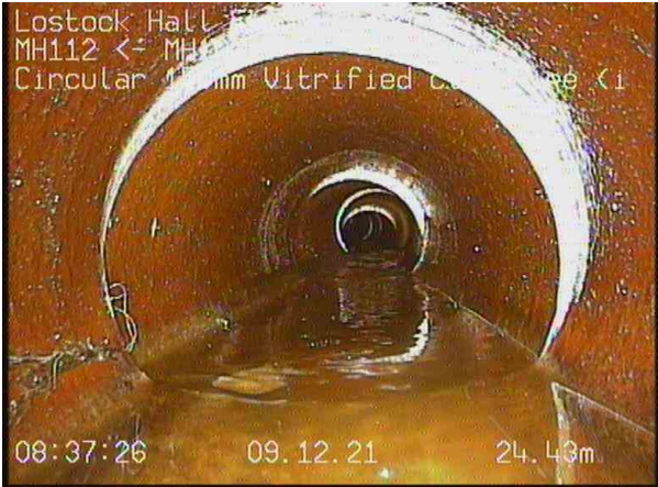
MH112X_f79f7a9b-4cf2-4bcb-8a14-13bd8f1be70c_20211209_084157_386.jpg, 00:04:09, 24.43 m Roots, fine at joint
