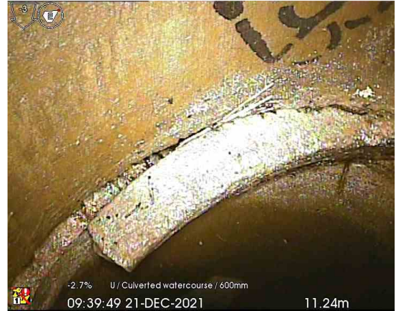
MH115X Overlap_11-24m_093949.jpg, 00:01:22, 9.75 m Fracture, circumferential at joint from 12 o'clock to 4 o'clock
