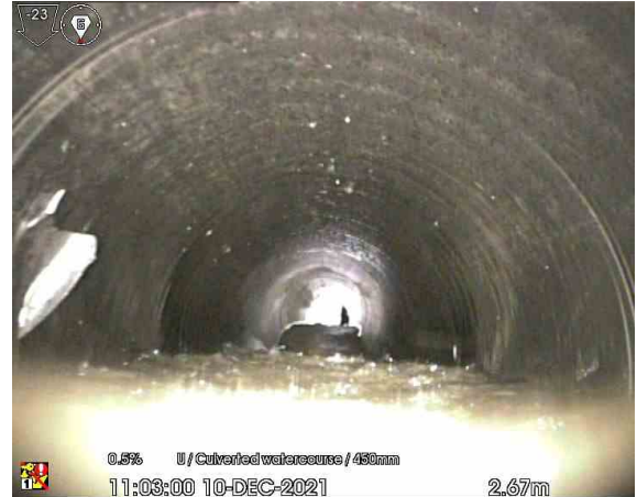
POND1X_2-67m_110300.jpg, 00:00:17, 2.67 m Surface damage, other from 9 o'clock to 10 o'clock, Surface damage, plastic has peeled.
