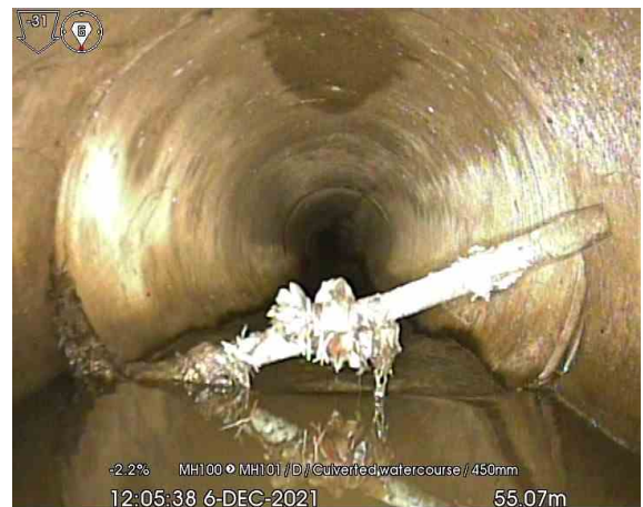
MH100X_55-07m_120538.jpg, 00:06:30, 55.07 m Survey abandoned, Unable to pass bar or branch with the crawler. Line needs jetting. TM needed.
