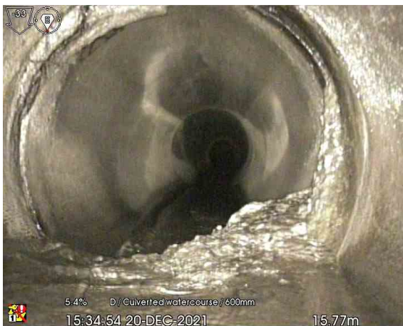
MH115X_15-77m_153454.jpg, 00:02:01, 15.77 m Survey abandoned, Risk to equipment. Survey overlapped from downstream manhole
