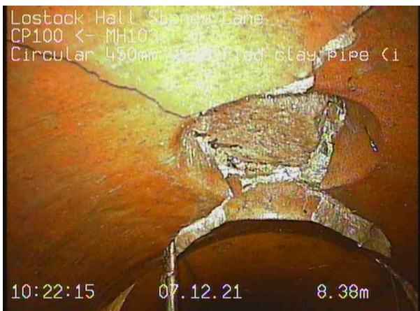
CP100X_c7afb641-09c1-4864-8684-5ba0da8ebdb5_20211207_092602_744.jpg, 00:02:17, 8.38 m Connection defective, connecting pipe is damaged at 12 o'clock, diameter: 150mm, Blocked and no sign of gullies within this area.
