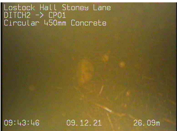
DITCH2X_d6608d2e-1516-4496-8d62-d7c5bf3b1b75_20211209_094817_724.jpg, 00:05:29, 26.09 m Roots, mass, 30% cross-sectional area loss
