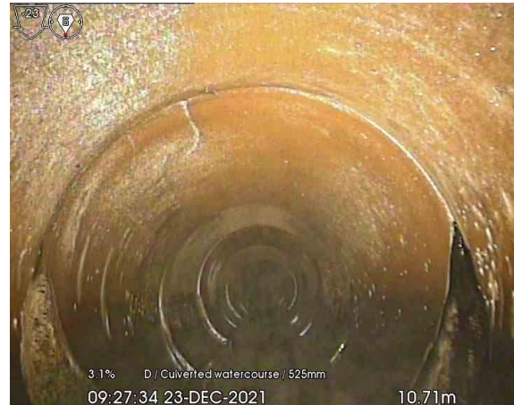
MH106X_10-71m_092734.jpg, 00:01:15, 10.71 m Crack, longitudinal at joint, at 11 o'clock
