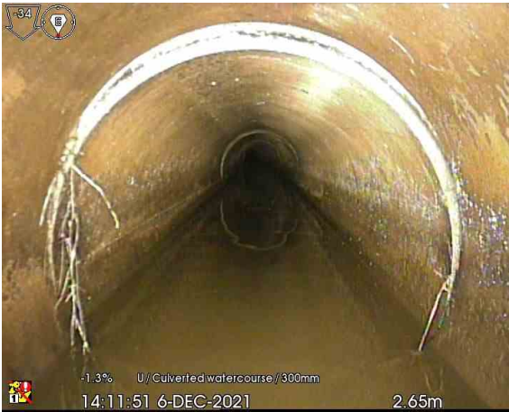
MH102X_2-65m_141151.jpg, 00:00:26, 2.65 m Roots, fine at joint
