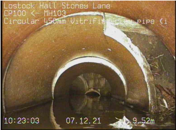
CP100X_df3e1c8c-c9c4-48ad-8804-7f15afaf9e4d_20211207_092650_656.jpg, 00:02:51, 9.52 m Hole in drain or sewer at a joint from 12 o'clock to 5 o'clock
