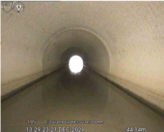
DITCH7X_44-14m_132923.jpg, 00:02:47, 44.14 m Settled deposits, fine, 20% % cross-sectional area loss
