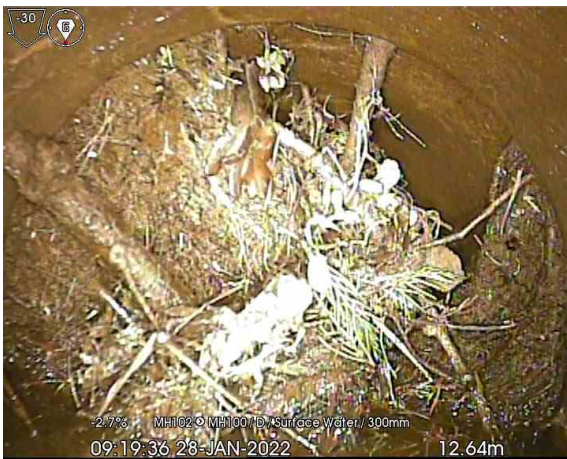
MH102X_12-64m_091936.jpg, 00:02:11, 12.64 m Survey abandoned, Unable to pass mass roots
