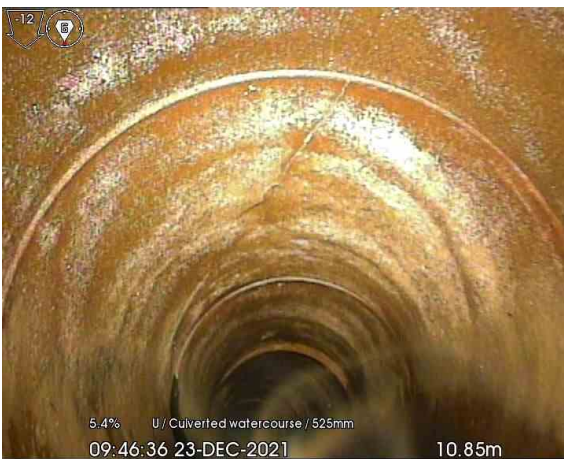
MH105X_10-85m_094636.jpg, 00:01:10, 10.85 m Crack, longitudinal at joint, at 12 o'clock
