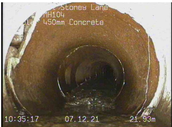
MH103X_13962f2c-f77b-473e-9097-880c88d8c147_20211207_093905_164.jpg, 00:02:15, 21.93 m Crack, circumferential at joint from 2 o'clock to 5 o'clock
