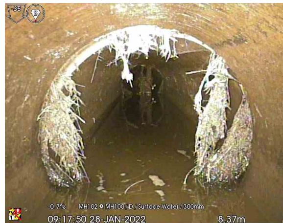
MH102X_8-37m_091750.jpg, 00:00:55, 8.37 m Roots, mass at joint, 30% % cross-sectional area loss
