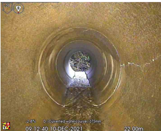
MH113X_22-00m_091240.jpg, 00:02:13, 22.00 m Crack, longitudinal at 3 o'clock
