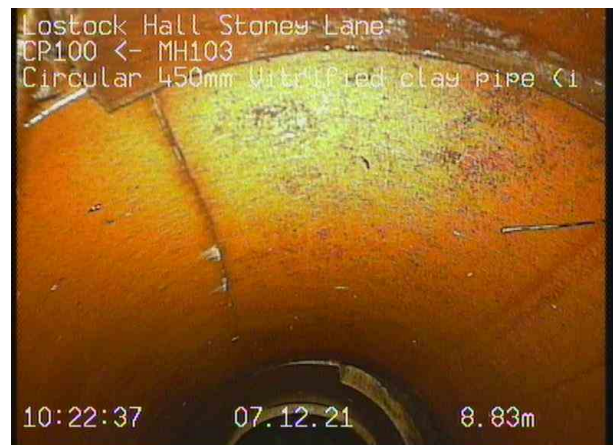
CP100X_1e224d9e-405b-47da-9010-a4eba253f7df_20211207_092624_848.jpg, 00:02:35, 8.84 m Crack, longitudinal at joint at 11 o'clock
