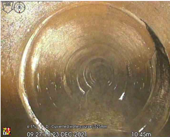
MH106X_10-45m_092718.jpg, 00:01:07, 10.45 m Crack, longitudinal at joint, at 03 o'clock
