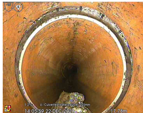
MH3X_17-77m_140559.jpg, 00:02:26, 17.77 m Open joint, medium
