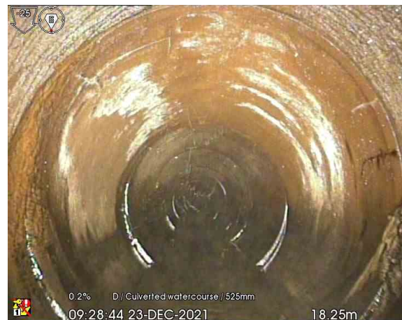
MH106X_18-25m_092844.jpg, 00:02:09, 18.25 m Crack, longitudinal at joint, at 03 o'clock
