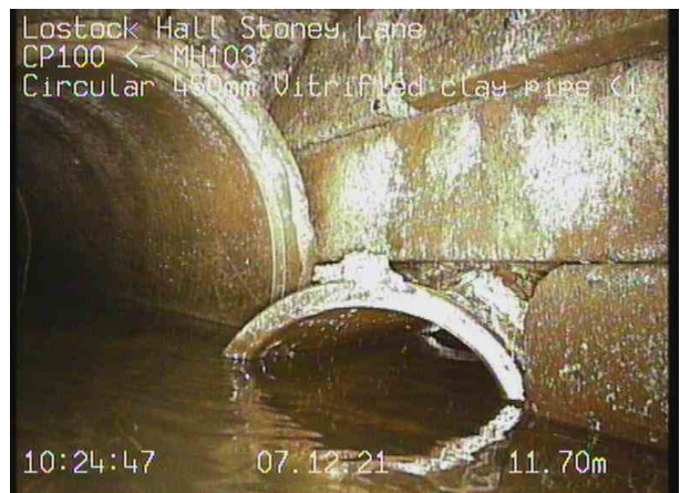
CP100X_562dccc1-b2f1-4f6c-9112-ebdc9effc733_20211207_092834_668.jpg, 00:04:00, 11.70 m General remark, Connecting pipe you can see in the catchpit is coming from Ditch1.
