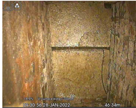
MH102 Upstream_46-34m_093056.jpg, 00:05:30, 46.34 m Finish node type, catchpit, reference number: Buried Catchpit, Buried Catchpit. Unable to continue survey as the crawler is dropping into a deeper section of the catchpit which will stop us from getting the crawler back.
