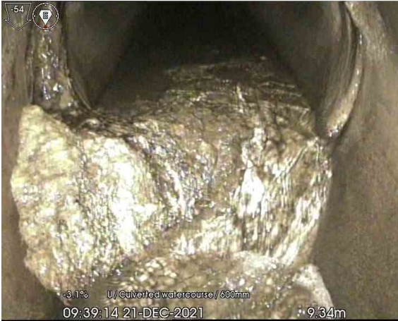
MH115X Overlap_9-34m_093914.jpg, 00:00:56, 9.34 m Attached deposits, encrustation at joint, from 04 to 08 o'clock, 20% % cross-sectional area loss
