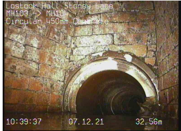
MH103X_b5c347e8-b384-42f1-8679-d35a71203a3c_20211207_094324_901.jpg, 00:06:10, 32.56 m Finish node type, catchpit, reference number: MH104, Buried
