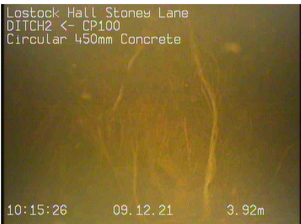
DITCH2X_82ea87bd-8f82-42f0-ae60-59e618eb32d9_20211209_101957_683.jpg, 00:01:32, 3.92 m Roots, tap
