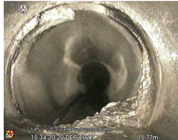
MH115X_15-77m_153420.jpg, 00:01:52, 15.77 m Fracture, circumferential at joint, from 09 to 12 o'clock
