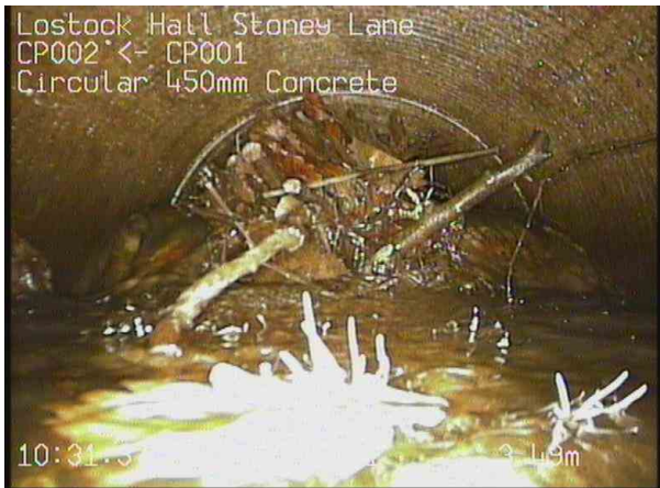
CP002X_0658fe4e-c858-4465-9642-e41be5d5b39a_20211207_103610_514.jpg, 00:00:27, 3.49 m Roots, mass, 90% cross-sectional area loss, Before Root-Cutting/Warthog
