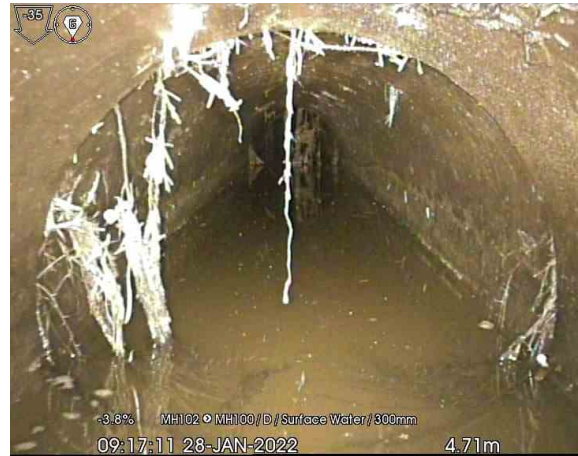
MH102X_4-71m_091711.jpg, 00:00:38, 4.71 m Roots, fine at joint
