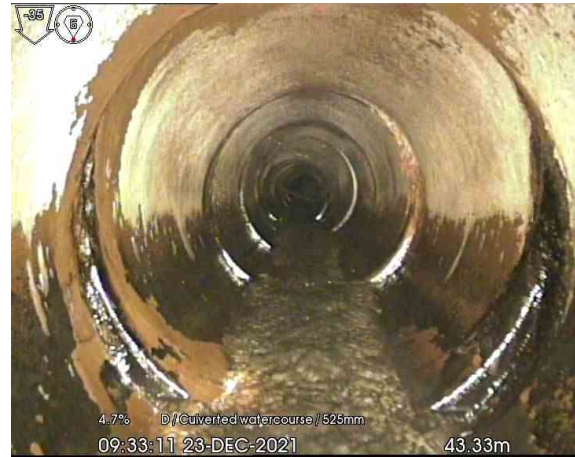
MH106X_43-33m_093311.jpg, 00:06:01, 43.33 m Infiltration, running at joint, from 11 to 05 o'clock
