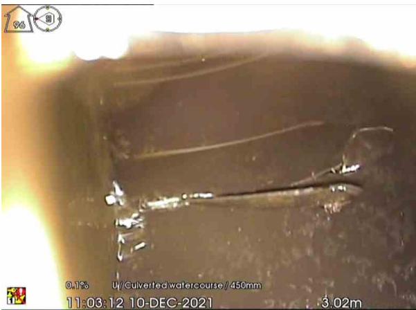
POND1X_95365508-cc5d-44a3-a42a-f720754d5abd_20220105_092539_965.jpg, 00:00:17, 2.67 m Surface damage, other from 9 o'clock to 10 o'clock, Surface damage, plastic has peeled.
