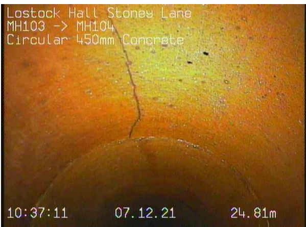
MH103X_f7c38e15-932b-42d6-95a7-6f00c36d977e_20211207_094059_279.jpg, 00:03:56, 24.81 m Crack, longitudinal at joint at 12 o'clock
