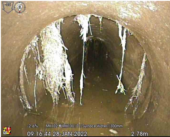
MH102X_2-78m_091644.jpg, 00:00:23, 2.78 m Roots, mass at joint, 20% % cross-sectional area loss
