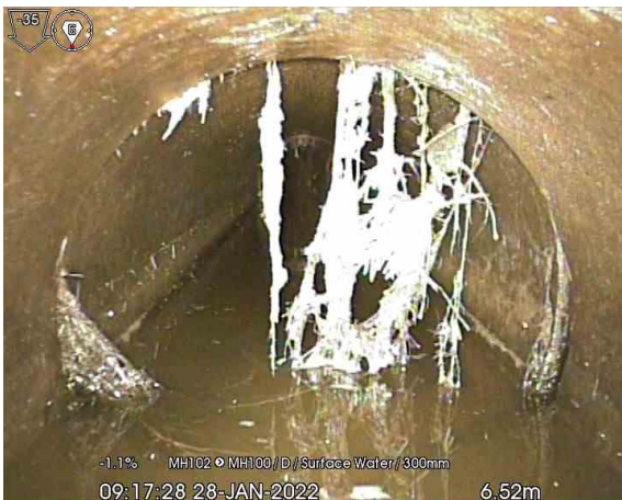
MH102X_6-52m_091728.jpg, 00:00:47, 6.52 m Roots, mass at joint, 20% % cross-sectional area loss
