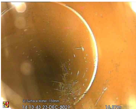
CP3 PIPE A_16-87m_141343.jpg, 00:01:39, 16.87 m Roots, fine
