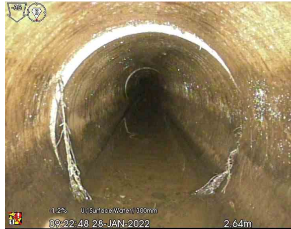
MH102 Upstream_2-64m_092248.jpg, 00:00:20, 2.64 m Roots, fine at joint
