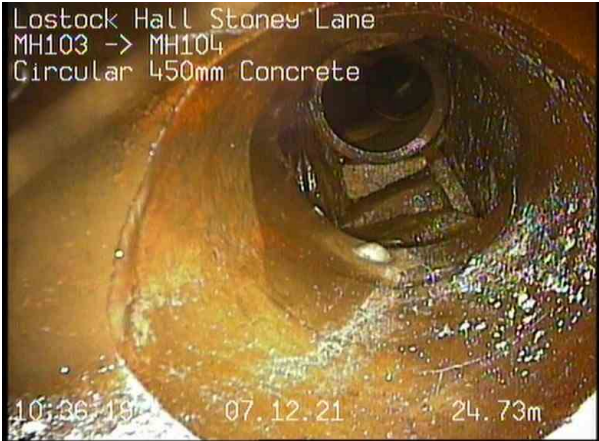
MH103X_0716da10-5474-4107-83a4-ac1df9286f47_20211207_100925_459.jpg, 00:02:50, 23.07 m Junction at 9 o'clock, diameter: 150mm, GY1
