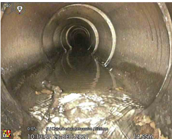
MH104X_14-55m_101327.jpg, 00:04:38, 14.55 m Survey abandoned, Unable to drive over rocks stuck on the joint. Line needs jetting. TM needed.
