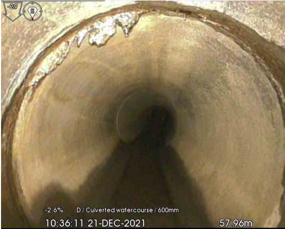
MH117X_57-96m_103611.jpg, 00:04:56, 57.96 m Attached deposits, encrustation at joint, from 10 to 12 o'clock, 5% % cross-sectional area loss
