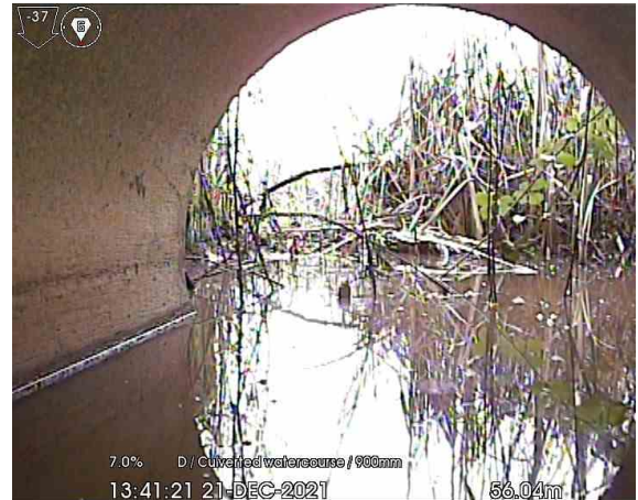
DITCH7X_56-04m_134121.jpg, 00:13:47, 56.04 m Finish node type, outfall, reference number: DITCH3, Ditch needs devegetation to drop the water level
