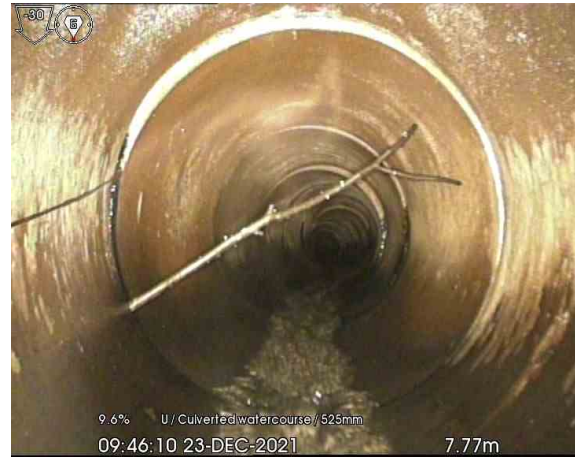
MH105X_7-77m_094610.jpg, 00:00:53, 7.77 m Roots, tap at joint
