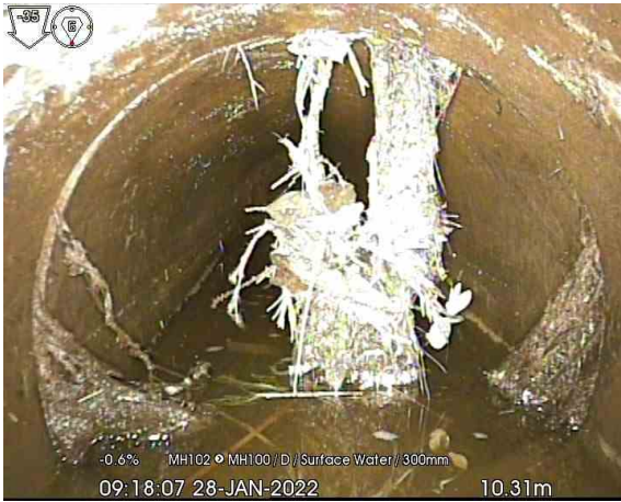
MH102X_10-31m_091807.jpg, 00:01:05, 10.31 m Roots, mass at joint, 30% % cross-sectional area loss
