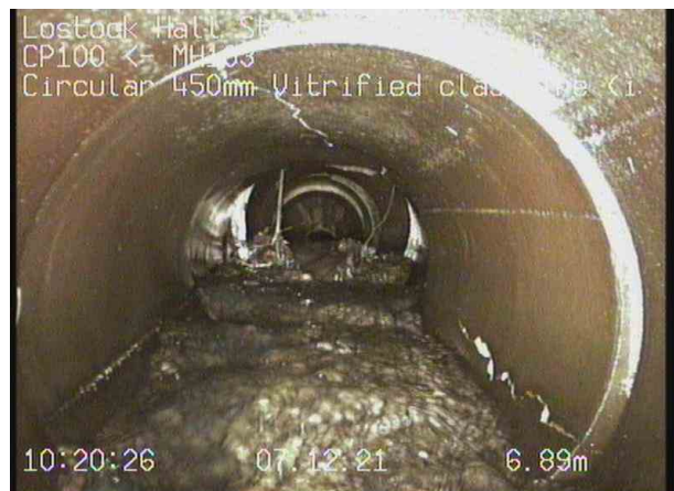
CP100X_d7148160-df8a-465f-bacd-fba022c64dea_20211207_092413_981.jpg, 00:01:14, 6.92 m Crack, longitudinal at joint at 11 o'clock
