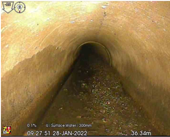
MH102 Upstream_36-34m_092751.jpg, 00:03:55, 36.34 m Settled deposits, fine, 20% % cross-sectional area loss
