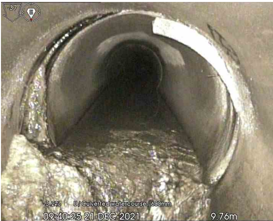
MH115X Overlap_9-76m_094025.jpg, 00:01:45, 9.76 m Survey abandoned, Survey overlapped from upstream manhole
