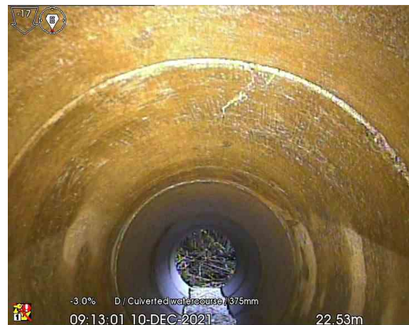
MH113X_22-53m_091301.jpg, 00:02:28, 22.53 m Crack, longitudinal at joint, at 12 o'clock
