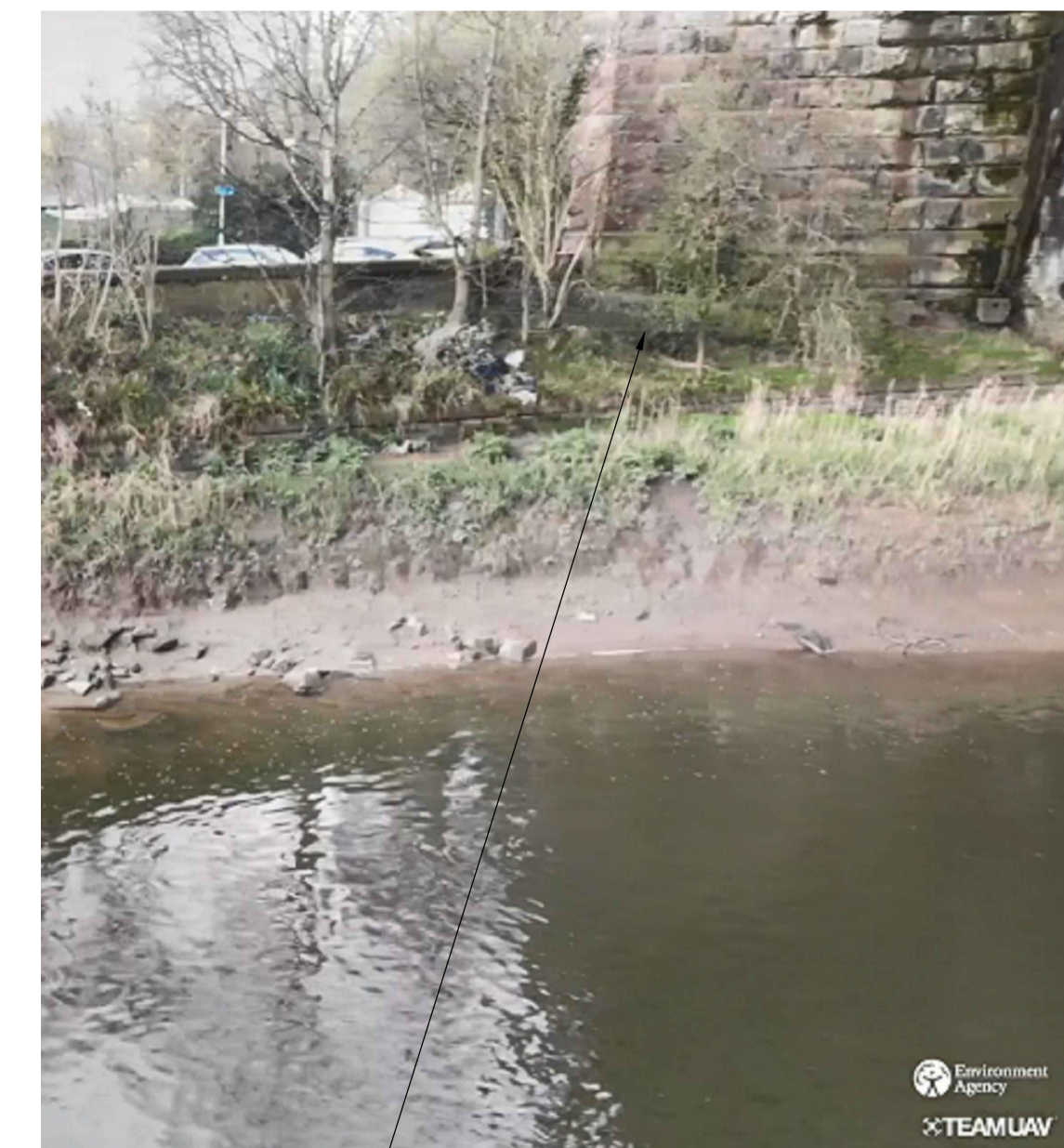
Existing channel bank in front of existing west coast main line railway abutment. Tie-in point for new Redi-Rock channel bank stabilization.
