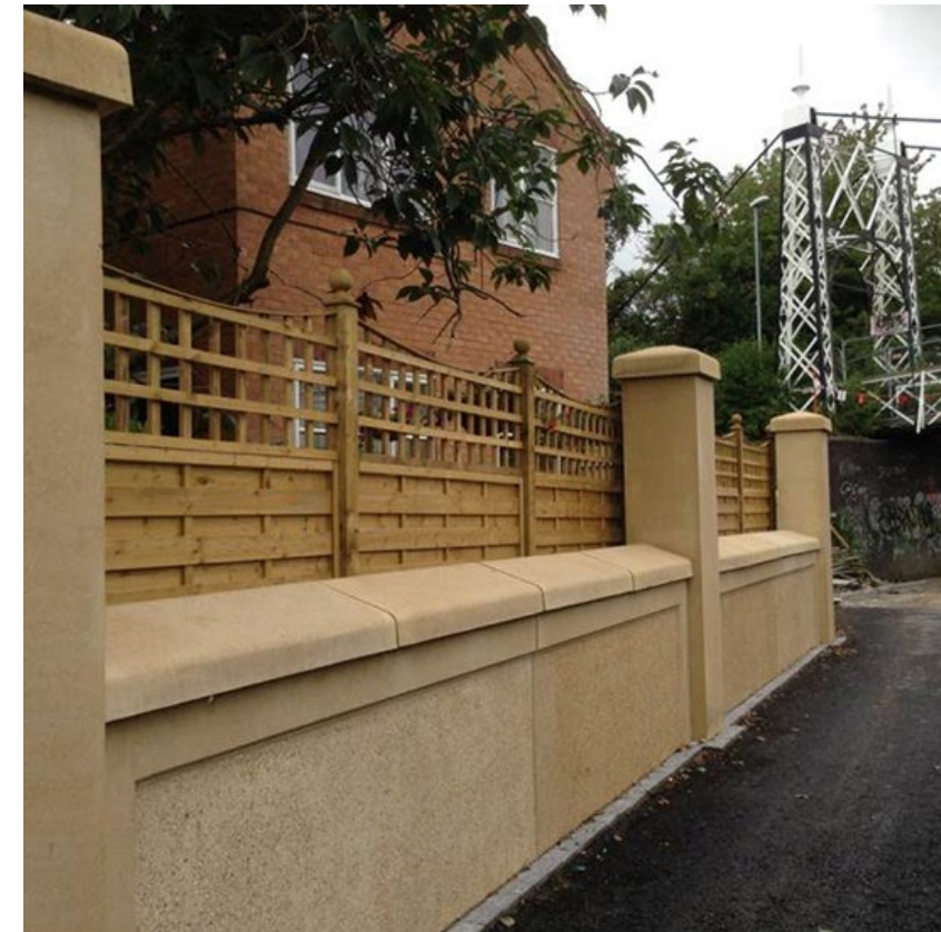
Example of flood wall with smooth picture frame and exposed aggregate centre.
