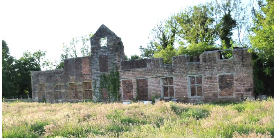
The Grade II listed ruin of an earlier Lower Hall dating from 1623
