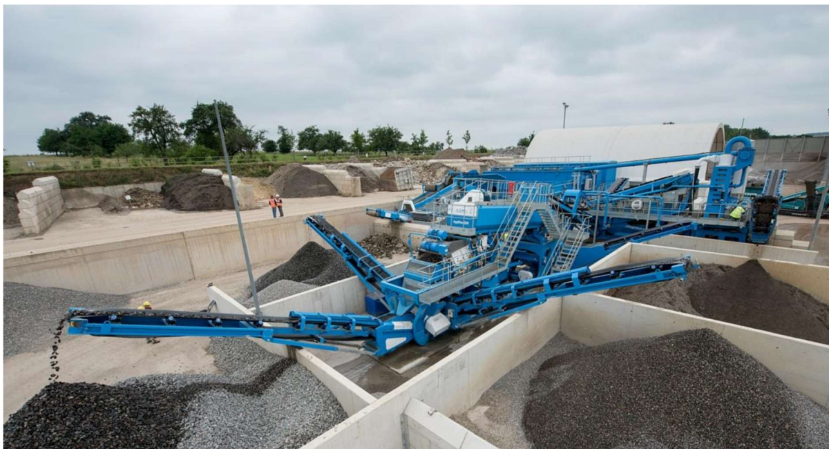
Figure 3.0 – Example Aggregate Wash Plant
