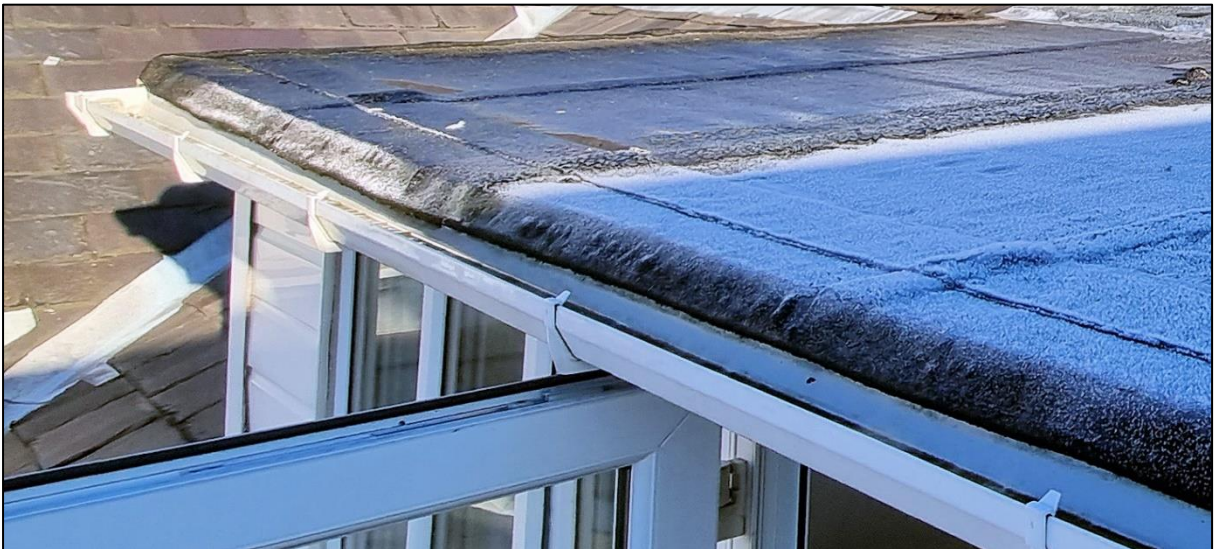
Plate 2: The roofing felts were intact with no gaps suitable for bats.
