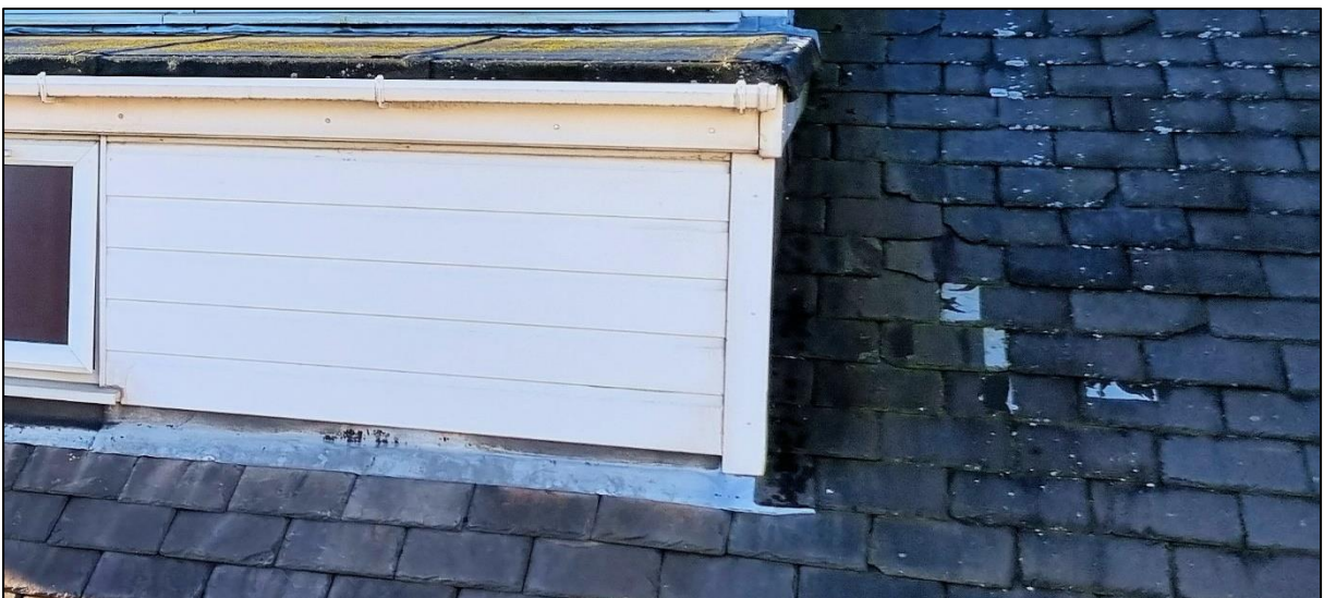
Plate 3: The cladding of the dormers had no gaps and no potential for bats.
