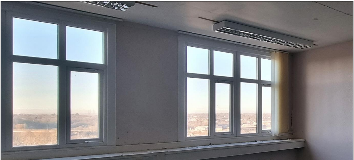
Plate 8: The windows of the dormers were intact with no potential access from the outside for bats.
