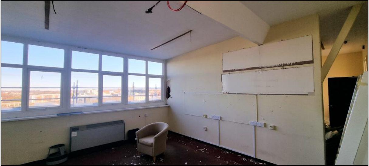
Plate 4: The offices in Zone A were open to the plaster board on the underside of the dormer roof.
