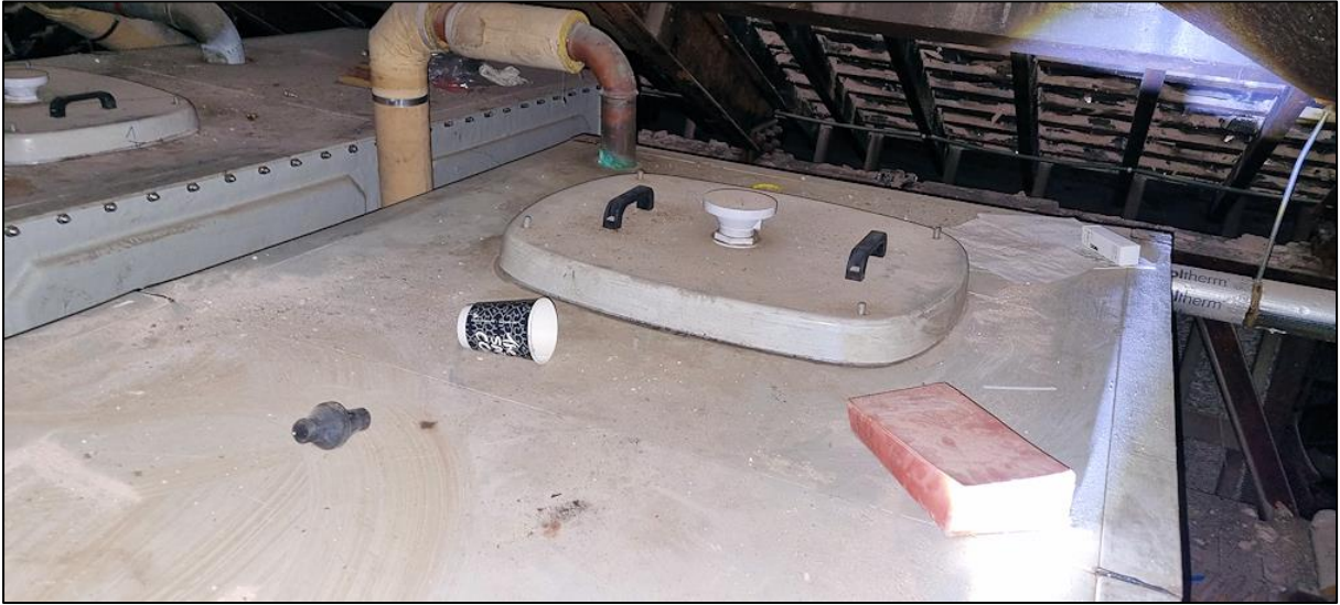
Plate 13: There was no evidence on the flat surfaces within the adjacent roof voids.
