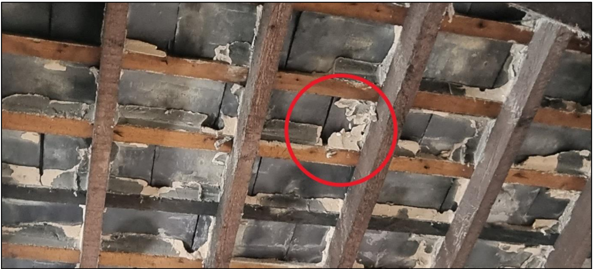
Plate 11: Where the mortar was missing there was potential access from outside the roof.
