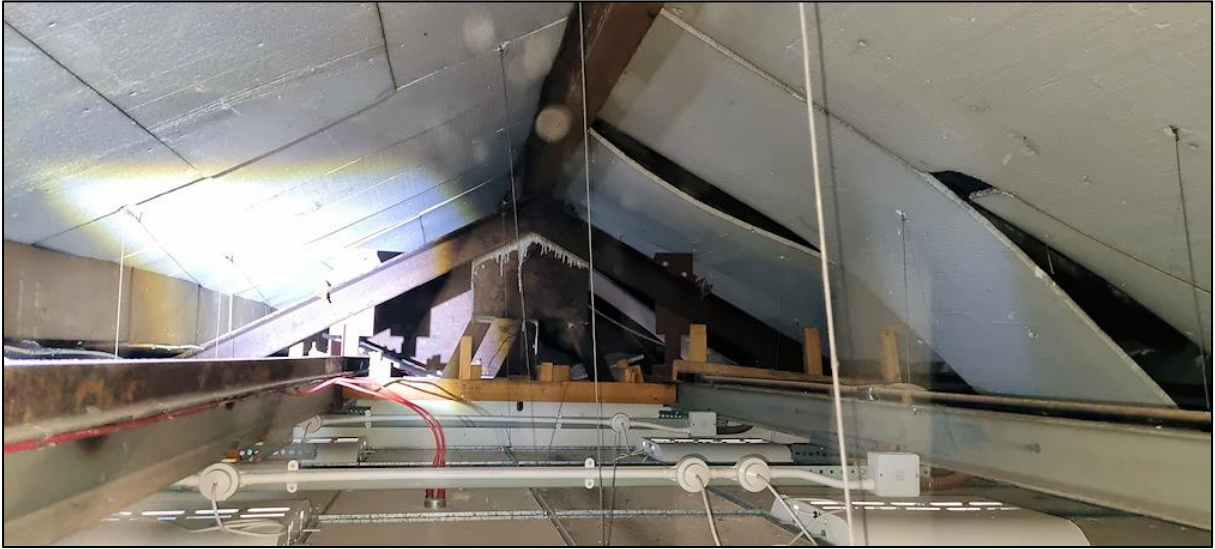
Plate 7: The void above the suspended ceiling in Zone B was partially boarded preventing inspection of the underside of the roof.
