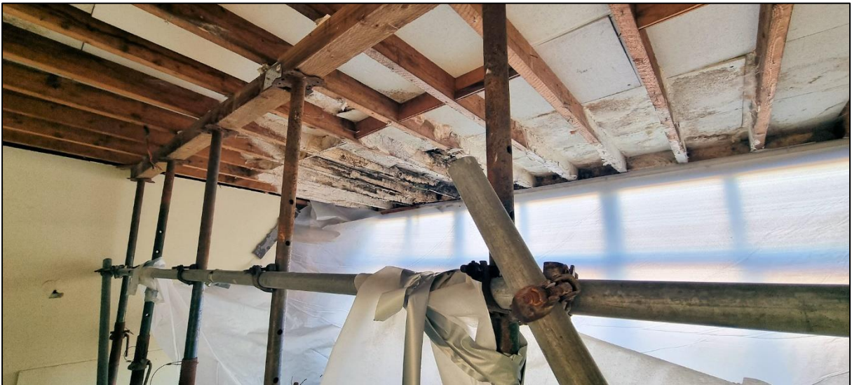
Plate 5: Where the plaster boarding had been removed the water damage to the timbers was apparent – there were no bat roosting opportunities here.
