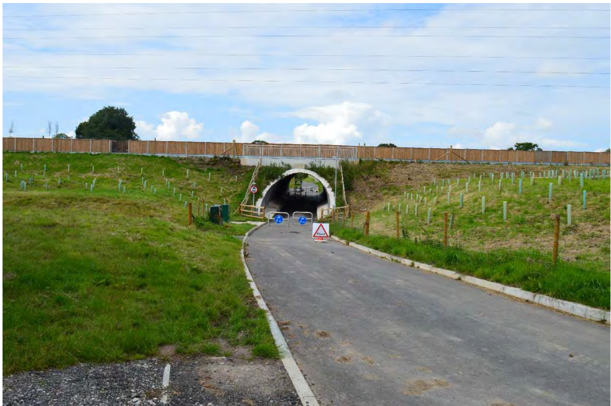
Plate 28: Area of disturbance south and north of Darkinson Lane, facing west
